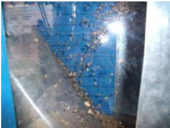
Figure 13. Grain screening inside the screening chamber.
